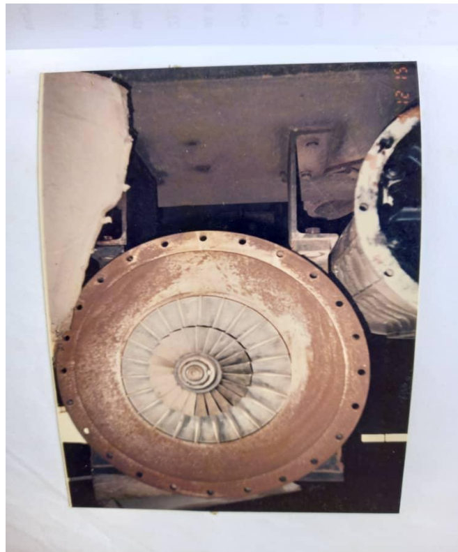
Fig.3: Corrosion in turbocharger assembly
