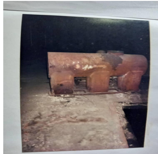
Fig. 6: Corrosion in exhaust manifold
